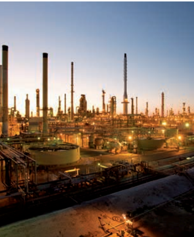
The 180,000 bpd refinery expansion at Garyville was approximately 75 percent complete at year-end 2008, with an on-schedule start-up expected in the fourth quarter of 2009.
